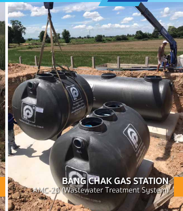
PTT GAS STATION AMX-2.5-40 (Wastewater Treatment System)
